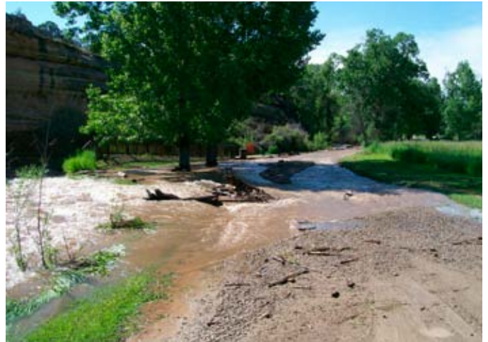
Medicine Lodge flooding, road washed away
